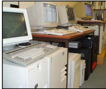
Disaster recovery & support systems, within our air-conditioned secure computer room at Cemoc House
